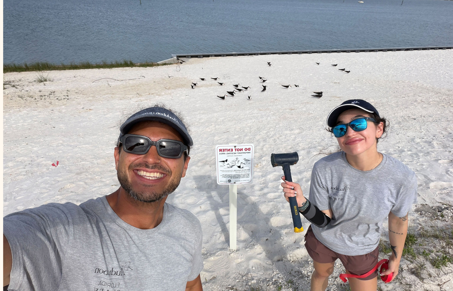
Audubon coastal team members Brian Cammarano and Alysia Martin install protective signs and fencing for a Black Skimmer colony nesting along the Navarre Bridge in the Florida Panhandle. Photo: Brian Cammarano/Audubon Florida.
